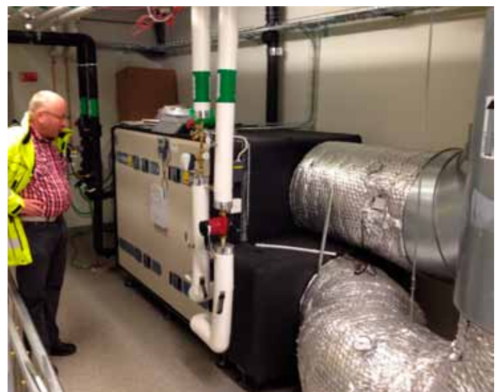
Technician Björn Adler inspecting a GOLD air handling unit. Photo: Swegon
